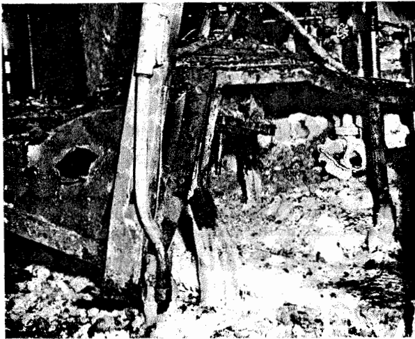
Figure 4. Close-up view of lower section of damaged pump area.
