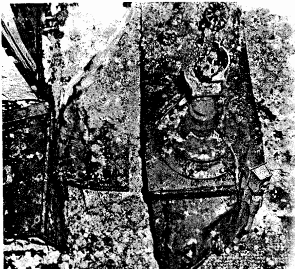
Figure 5. Overhead view taken from catwalk over Freon system of liquid oxygen pump area.
